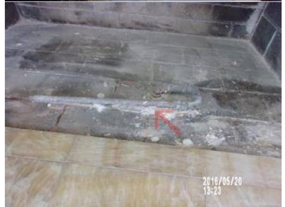
Gas pipe too close to the opening.
